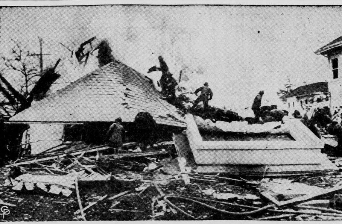
FIREMEN COMB THE WRECKAGE OF A TWO-STORY HOUSE in southwest Los Angeles for possible victims after the building was completely demolished by a violent explosion. Four exterminators were reported to have been inside the house when the blast occurred. Three of the men were injured.
