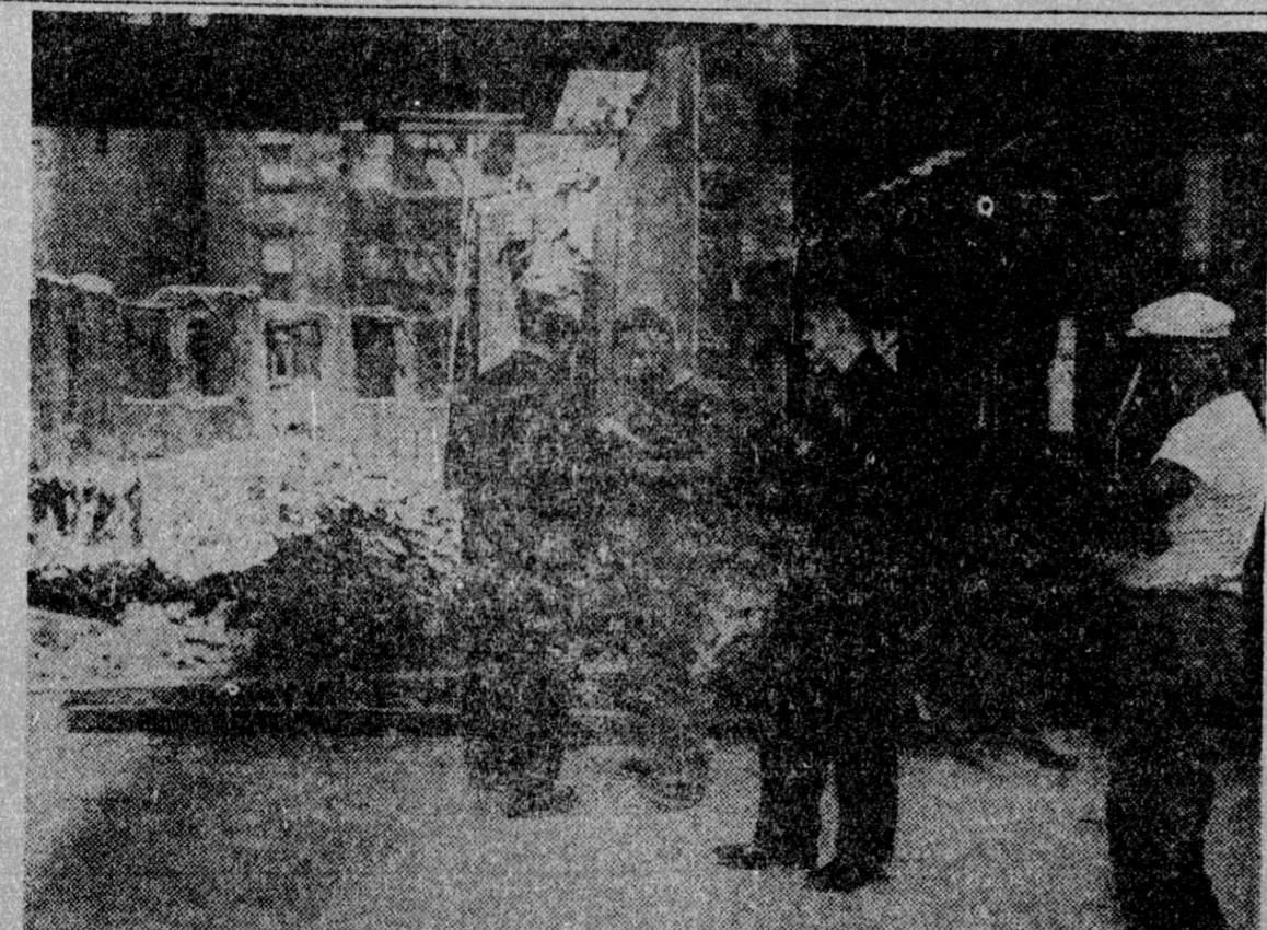
THE $60,000 QUESTION — During the recent demolition of five-story New York tenement, workmen uncovered a cache of $60,000 in $100 bills. Before the cops could act on an anonymous tip, several of the men had "done the town" with their findings. Here, foreman Michael Leach (short sleeve shirt) tells police what he knows about the treasure. If no one claims the loot in 90 days, the workman will share in what's left of the $60 grand. (NEWSPRESS PHOTO)
