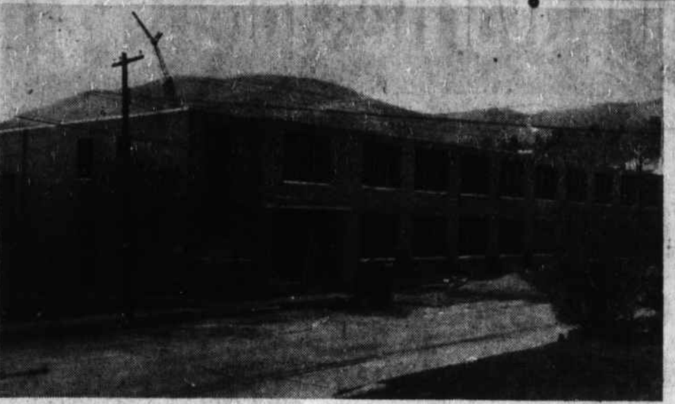
ELEMENTARY SCHOOL—Work progresses on the new Elementary School building being constructed here on College Street.—Staff photo by Joe Minor.
