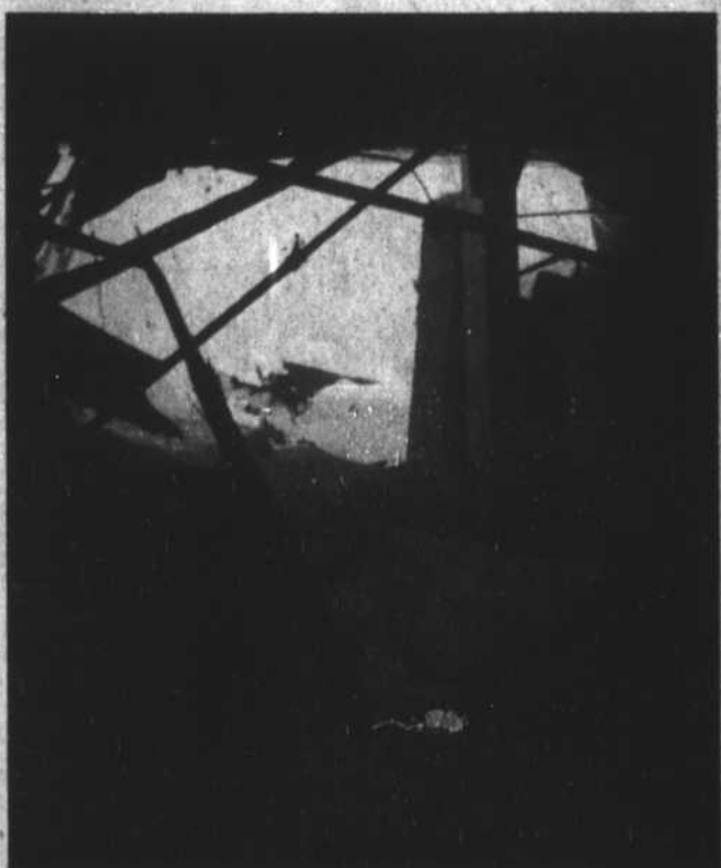
HOLE IN ROOF lets daylight shine through warehouse of Farmers Hardware and Supply Co., Inc., after drifting snow caused the roof to cave in last week. Twisted pipes, part of the sprinkler system, may be seen. The pipes, which were fed by a four-inch main, broke and spilled tons of water on merchandise stored there and on the floor of the building and into the street where it froze. Russell D. Hodges, Sr., president of the firm, said Tuesday that preliminary estimate of damage was placed at $5,000 to $7,000, but that exact figures would not be known until all damaged supplies could be moved. Work has been hampered by the freezing temperatures following the cave-in.—Staff photo.
