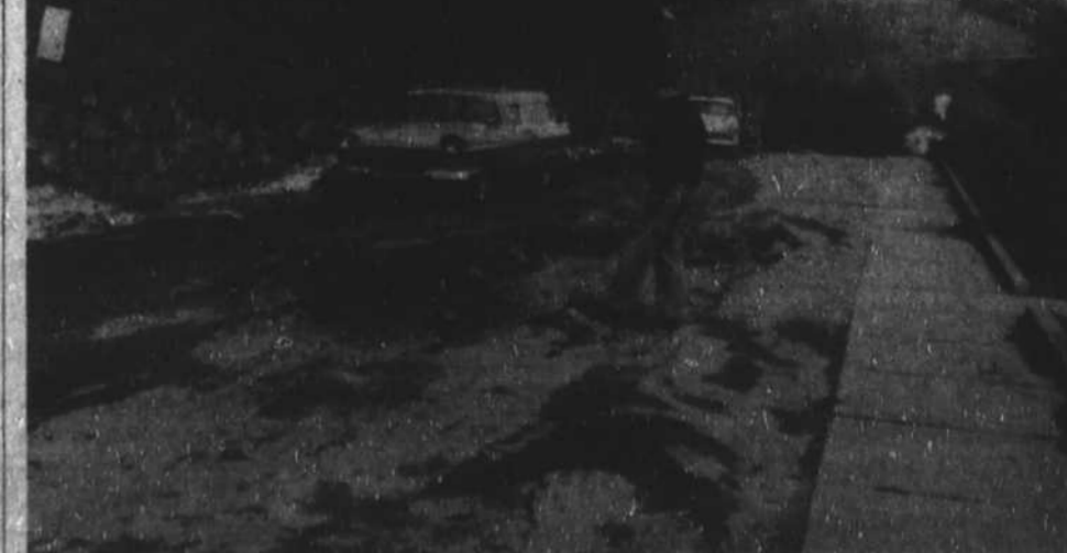
WINTER'S TOLL.—J. B. Robinson, Boone, examines hole in side street at postoffice which has cracked and broken, due to the hard freeze and quick thaw in this area. Other streets in town have suffered similar damage also, but most of them have remained passable to traffic. This street was closed after its sudden collapse and one car required wrecker service to get it moving after sinking into the soft dirt and broken asphalt.—Staff photo Joe Minor.
