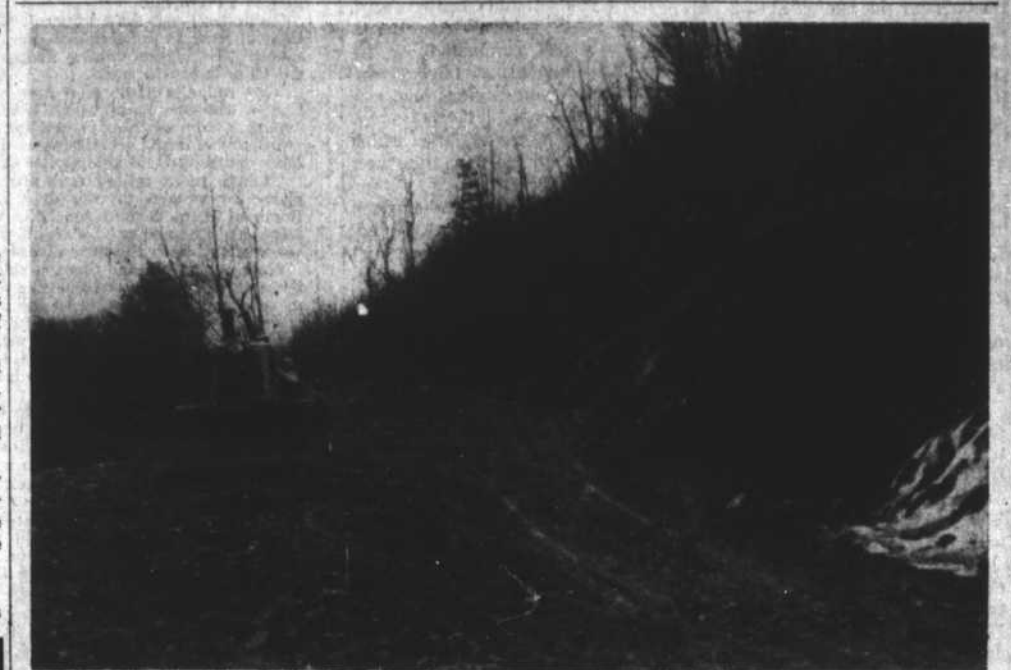
GOLF COURSE ROAD. —A bulldozer sits idle at the entrance of the Boone golf course, after pushing out a road into the development. The road was built in preparation to developing the project, beginning this spring. The course is located off the Blowing Rock highway, just out of Boone.—Staff photo.
