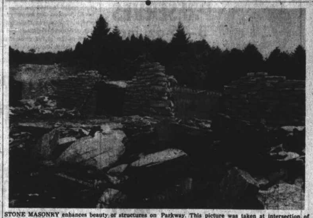
STONE MASONRY enhances beauty of structures on Parkway. This picture was taken at intersection of Scenic and Triplett Road, where overpass is being built.
