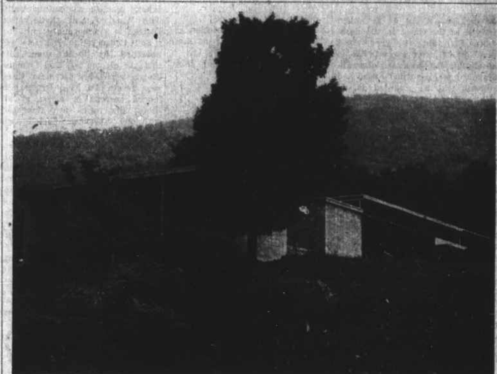
NEW COUNTY SCHOOL OFFICES AND GARAGE takes shape west of Boone just off Highway 421. The building is on the property formerly occupied by the old county home, and is next to the Health Department building. It is hoped the structure will be ready for occupancy sometime this fall.
