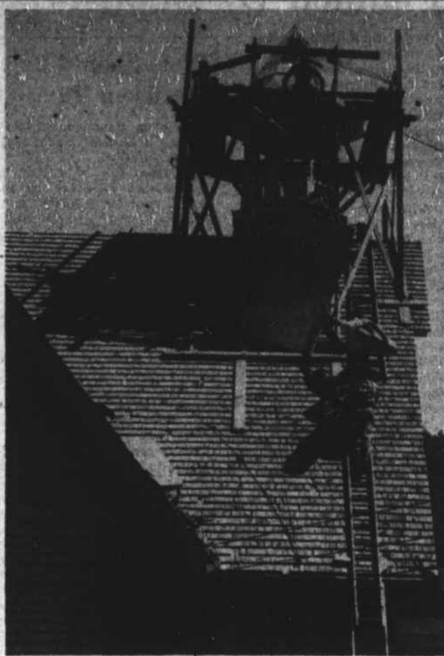
STEEPLE gets "new look."—Raymond Jones and crew of men, Ed Hayes, Bill Jones, and J. B. Greene, re-covered the steeple of Poplar Grove Baptist Church last week with a bright copper roofing. This is one of the projects started several years ago by the members in improving their church building. They have repainted the church, inside and out, installed a new heating system, and are getting ready to re-roof the building and enlarge and improve the parking lot. Several thousand dollars have been pledged to the improvement plan, according to a spokesman of the church.—Staff photo by Joe Minor.
