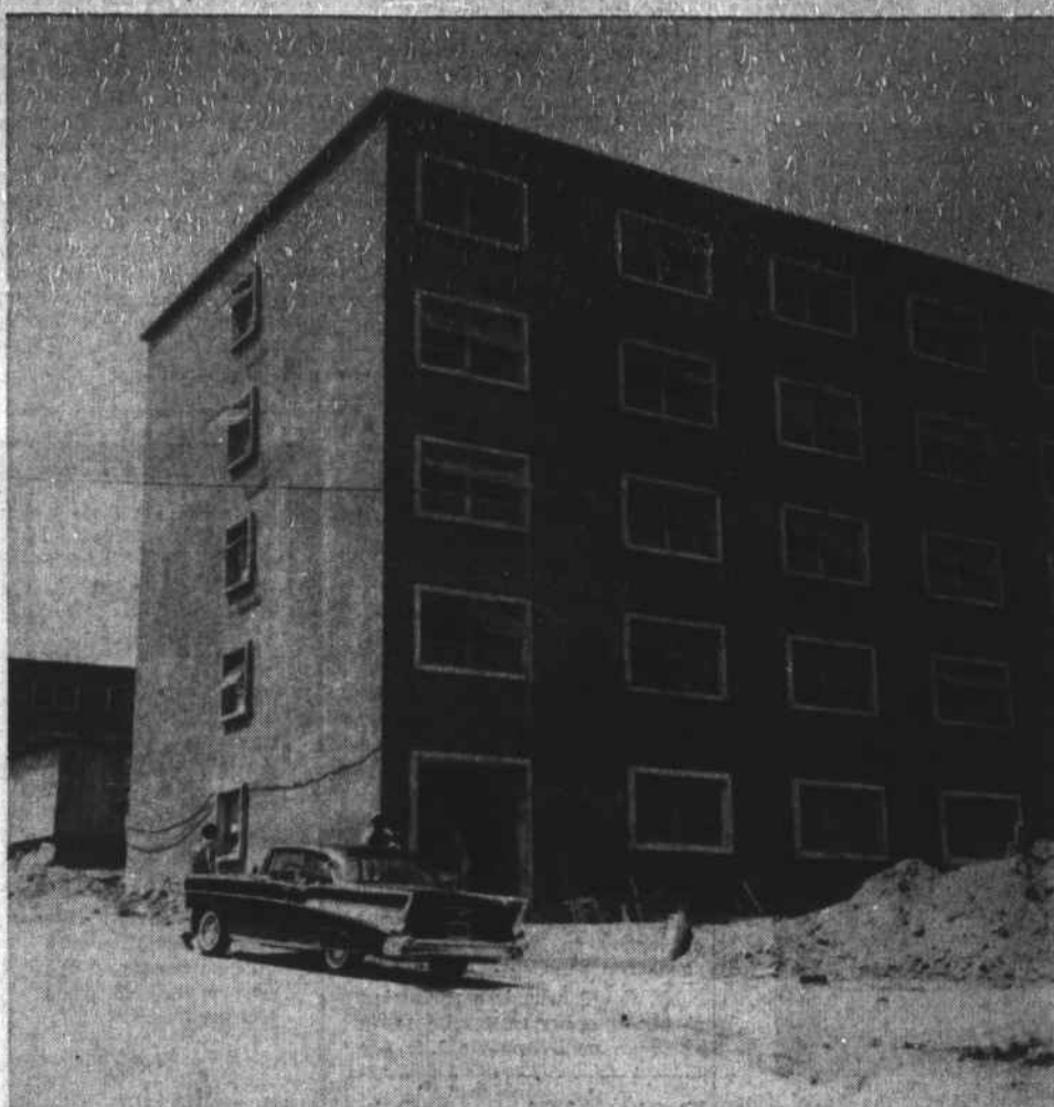
DORM NEARS COMPLETION.—The south-east end of the new wing of East Hall is nearing completion, and it is expected that it will be ready for occupancy when the fall term begins in September. The building will house 176 Appalachian girls when completed. See story on page two.
