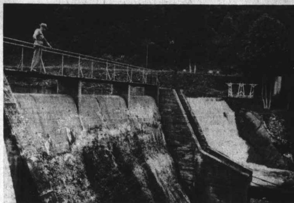
DAM DAMAGE.—S. M. Ayers, superintendent of New River Light and Power Company, surveys erosion and cracks in company's power dam which are to be repaired. The work will be done after sealed bids are opened September 17.—Staff photo Joe Minor.
