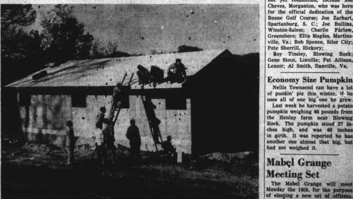
FINISHED NOW. —Carpentry students of Appalachian High School get actual training in building. This house has been completed and will be put up at auction Saturday morning. “Open House” Friday will precede the sale. (Story on page two, section B).—Photo by Verlin Coffey.
