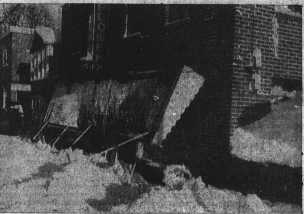
HEAVY SNOW.—The metal awning at Boone Flower Shop broke loose from its moorings late Saturday night from the weight of the week end snow. Mr. and Mrs. Harold Hartley, owners of the shop, were preparing to go home, and had already locked the doors and were cleaning the snow from their car when the awning fell. It was repaired and put back up Monday.—Staff photo.
