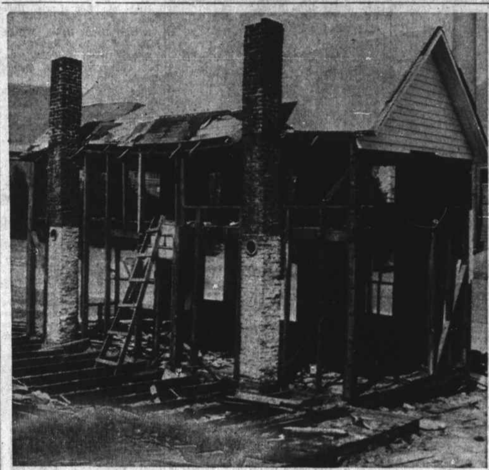
MAKING WAY FOR PROGRESS —One of two houses being removed from site where college's Home Economics building and Home Management House will be built. Work is expected to get underway on buildings this summer. Almost directly across Faculty Street from the Home Ec. buildings will be built an Industrial Arts plant. Work on this latter project is not expected to start until after the Home Ec. buildings are begun.
