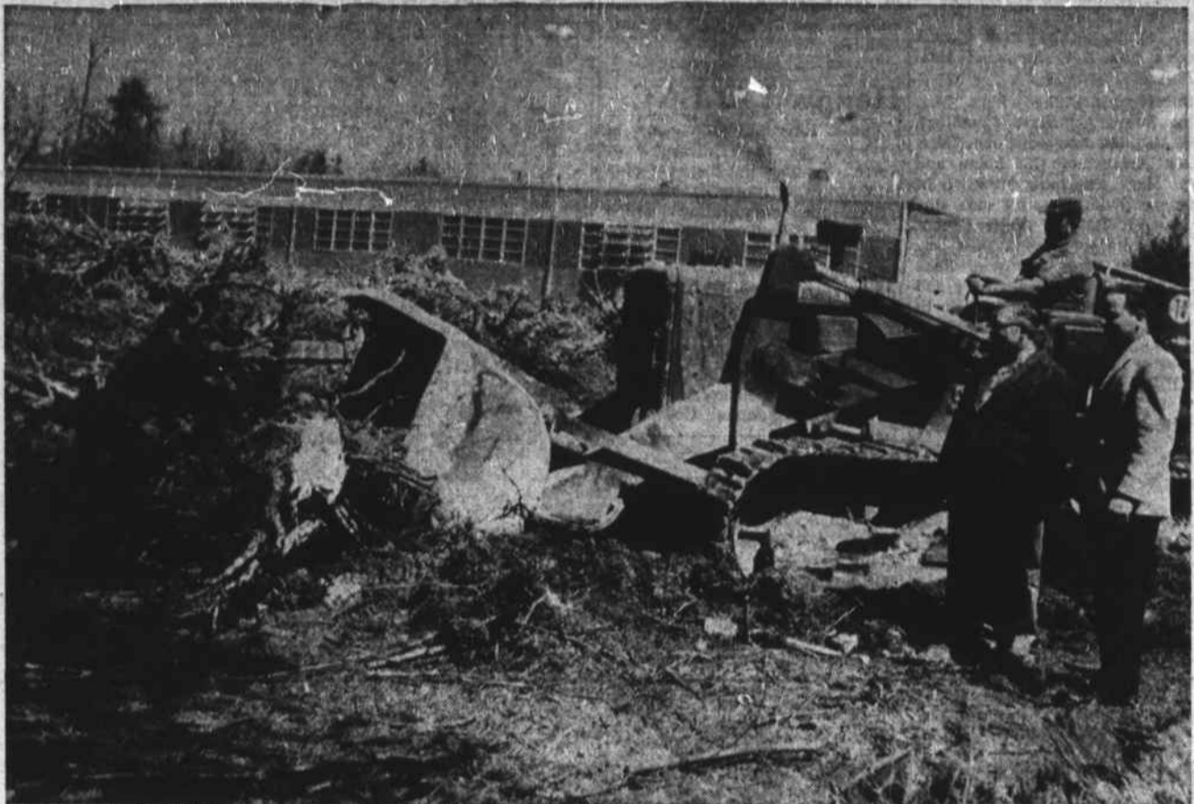
BUILDING SITE —Homer Shore operates bulldozer in stump field where addition to Shadowline plant will be built. Hubert Inman, plant engineer (left), and John D. Broyhill, administrative assistant, watch as the stumps are pushed from the ground.
