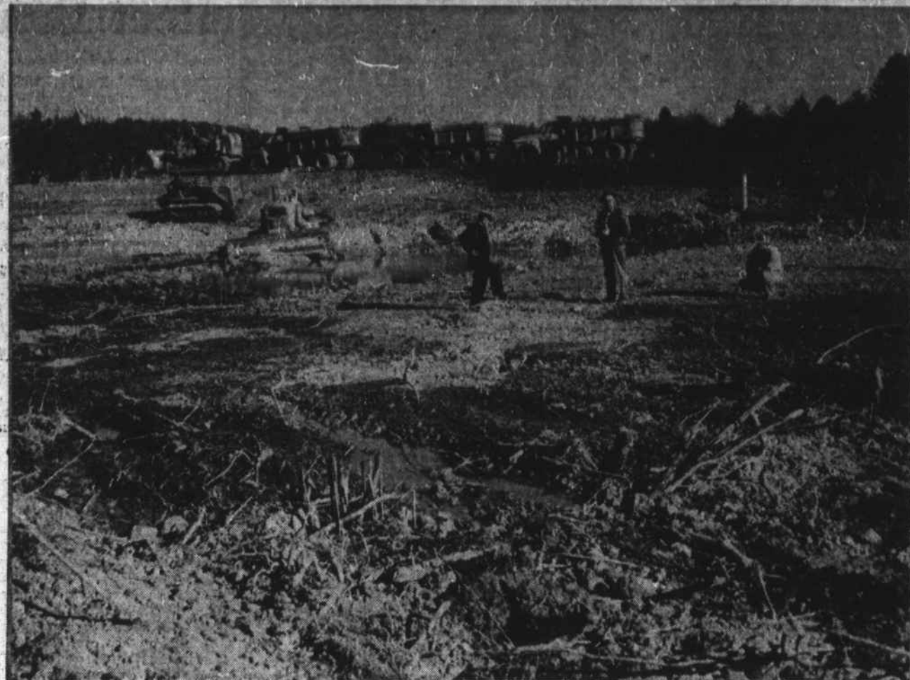
FUTURE FISHING.—Boone Chief of Police G. D. Richardson (left) talks with O. M. Hampton and Howard J. Williams about fishing ponds he is developing in the Ruthewood section. Bulldozers are clearing the land and building dam for one of three ponds the chief expects to stock with fish for public fishing.
