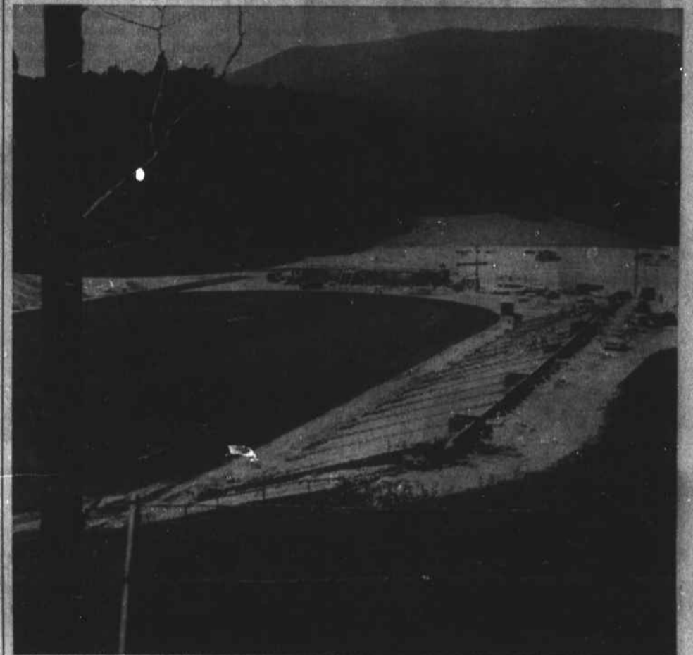
ASTC STADIUM construction continues through August as the opening date for the mammoth structure, hollowed out of a natural mountain basin, draws near. The first football game to be played on the new field is scheduled for September 15 when the Mountaineers face Emory and Henry. Advanced tickets will go on sale in the near future, according to a college spokesman. The above picture was taken from the upper rim of the stadium, looking northwest. The field house is in the background.—Photo by Gaddy.
