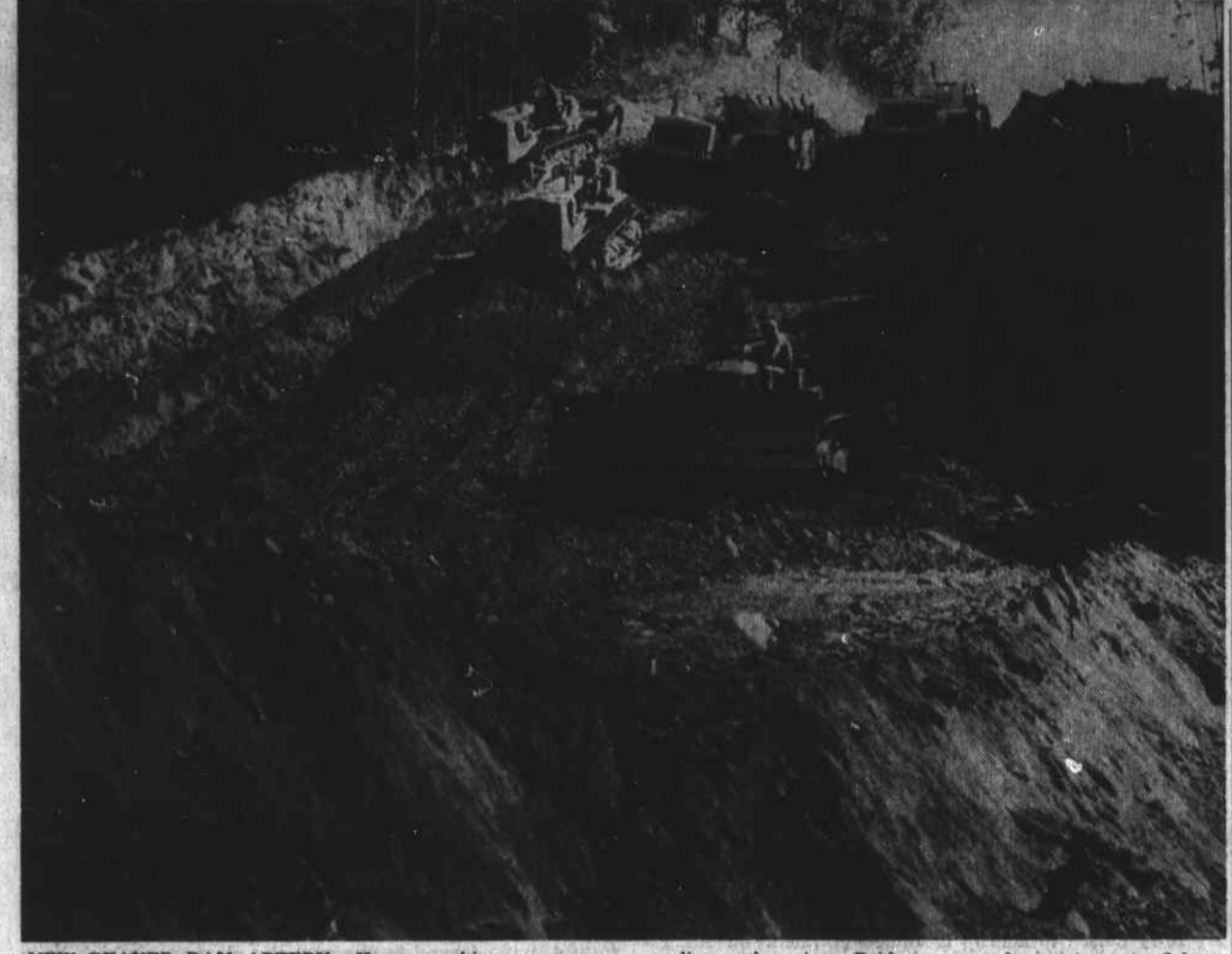
NEW BEAVER DAM ARTERY. —Heavy machinery moves dirt on new highway which leaves 421 near the Windy Gap Church and will extend 1.61 miles into Beaver Dam township. The cost of the project is given at $400,000, and the Sherman Simpson Co., of Mount Airy, has the contract for
