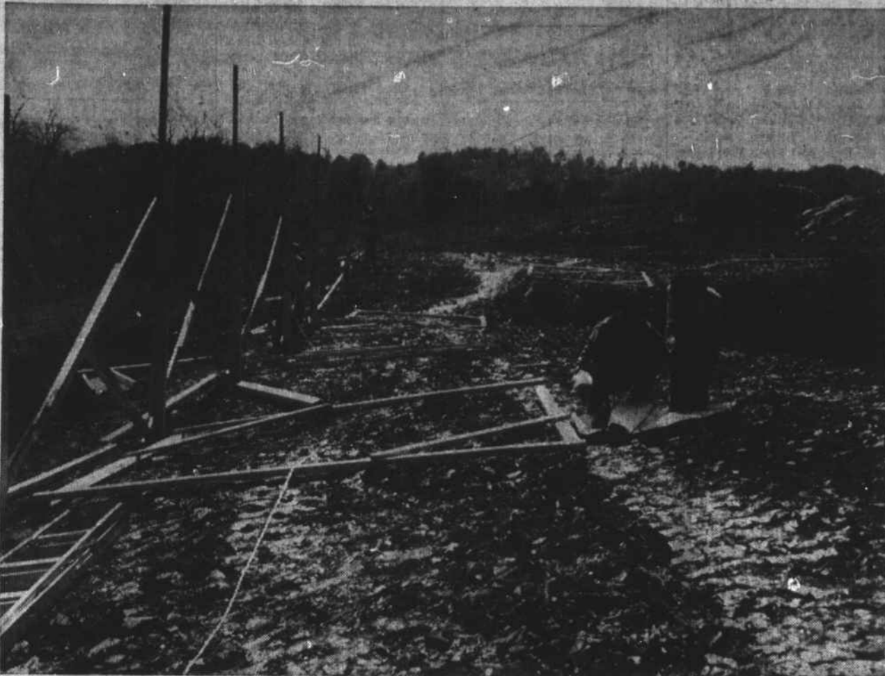
Grading has been finished for the new seven-story dormitory for women for Appalachian State Teachers College. Men are shown on the grade looking at plans for the structure which will cost $765,000 and which is scheduled to be ready
