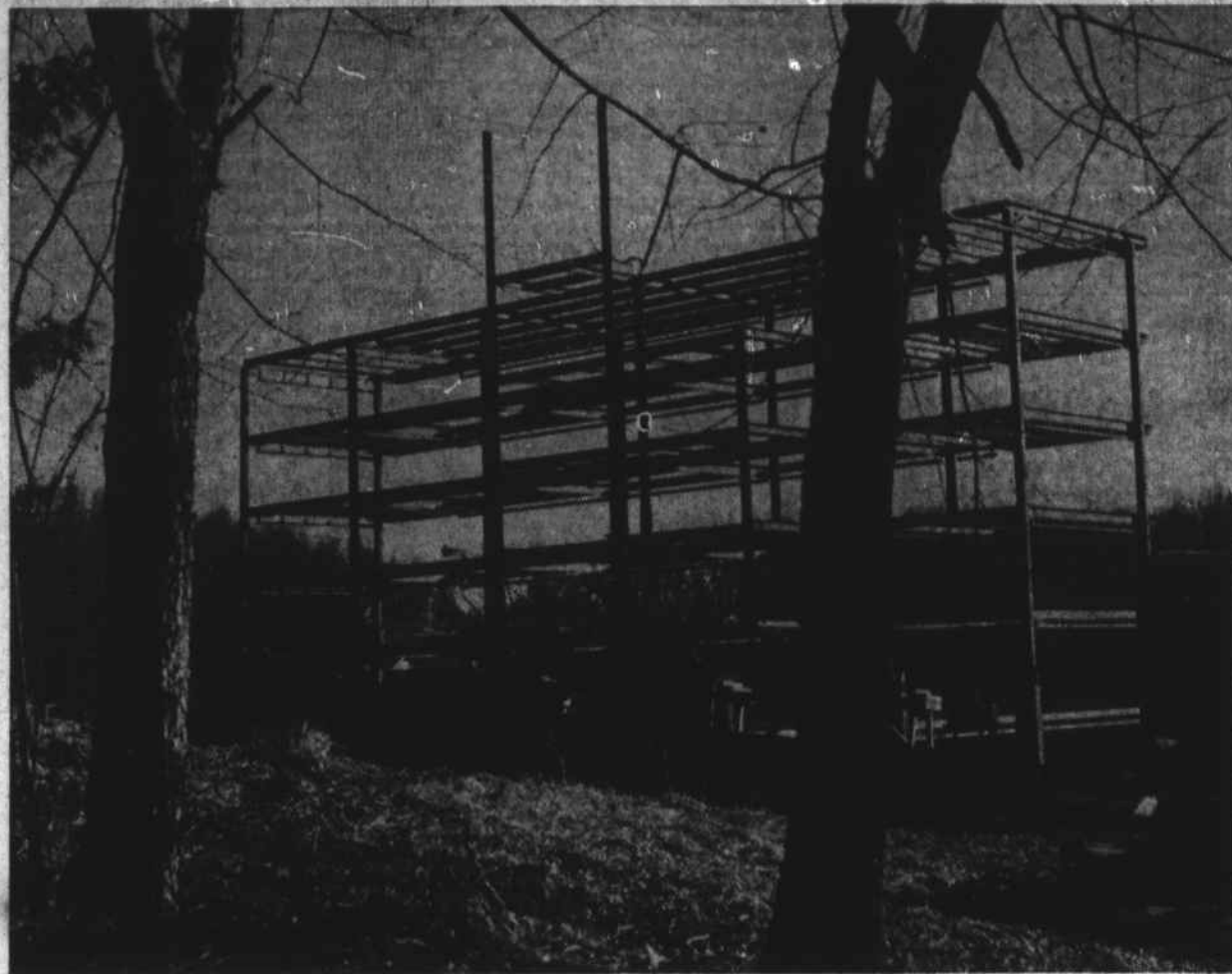
DORMITORY CONTINUES CLIMB. —The new seven-story girls dorm being constructed on the east edge of the ASTC campus spirals upward as work crews make progress in cold February winds. College officials are hoping the dorm will
