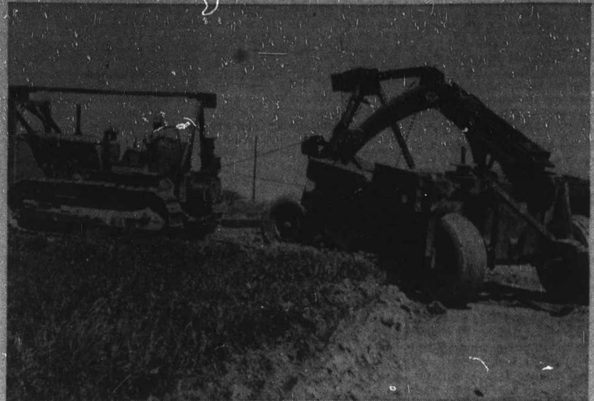
HEAVY EQUIPMENT IS SEEN MOVING DIRT at the site of Watauga County Hospital on Deerfield Road.
