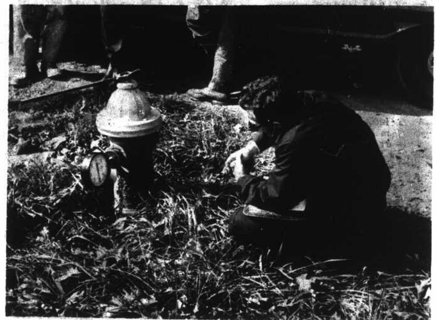
Soon after a water shortage was discovered Oct. 13, engineers began compiling information on water pressure at various points in Boone. Here, a man reads a gauge on Blowing Rock Road. Fluctuation of pressure was carefully noted as teams of men analyzed the crisis.
