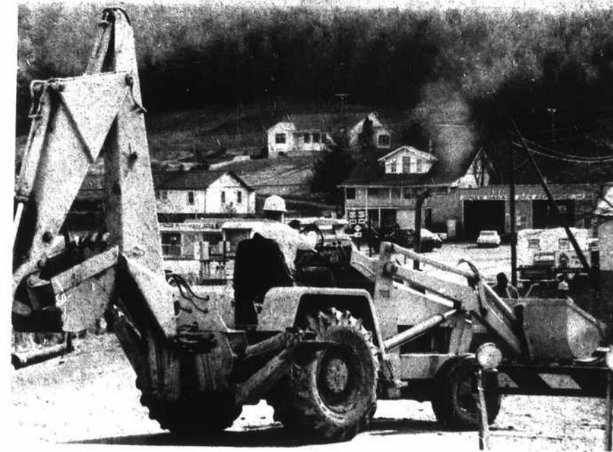
HEAVY MACHINERY IN PERKINSVILLE—Work on Boone's $1,860,000 water-sewer project is underway in Perksville, which was annexed with two other outlying districts when the city voted the bonds. Flagmen are
