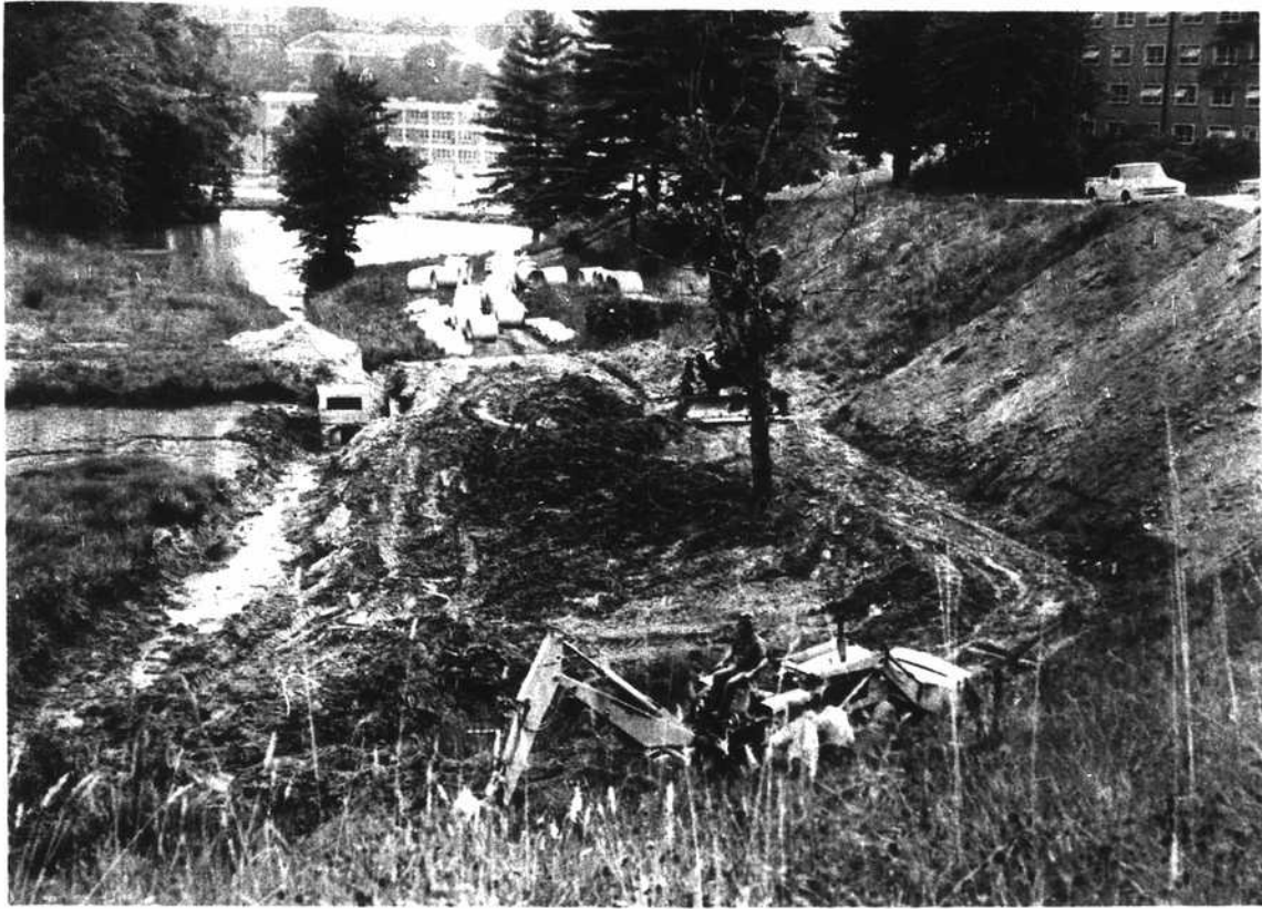
A RECREATION AREA is being created for a men's dormitory being constructed near Conrad Stadium on the ASU campus. When the ravine is filled in, additional space will also be provided for parking during football games. The campus pond (background) will not be covered at the present time. (Staff photo)
