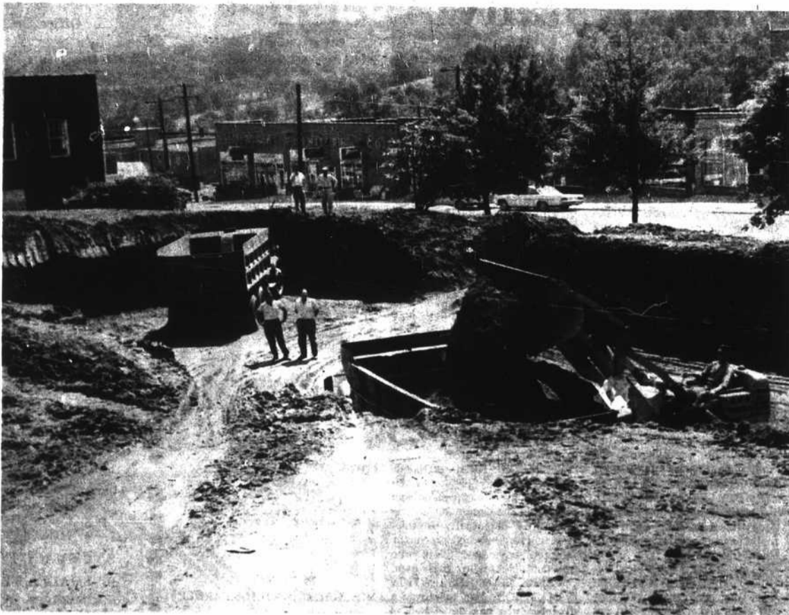
AT THE SITE OF THE NEW COURTHOUSE, dirt-moving machinery hollows out a space for the vault, in which County records are to be stored. With good weather, the building contractor planned to pour the footings for the modern structure this week. The $450,000 project is to be completed within 12 months. A basement will be sunk at the back of the site (to the left of this shot) to contain the boiler room. (Staff photo)
