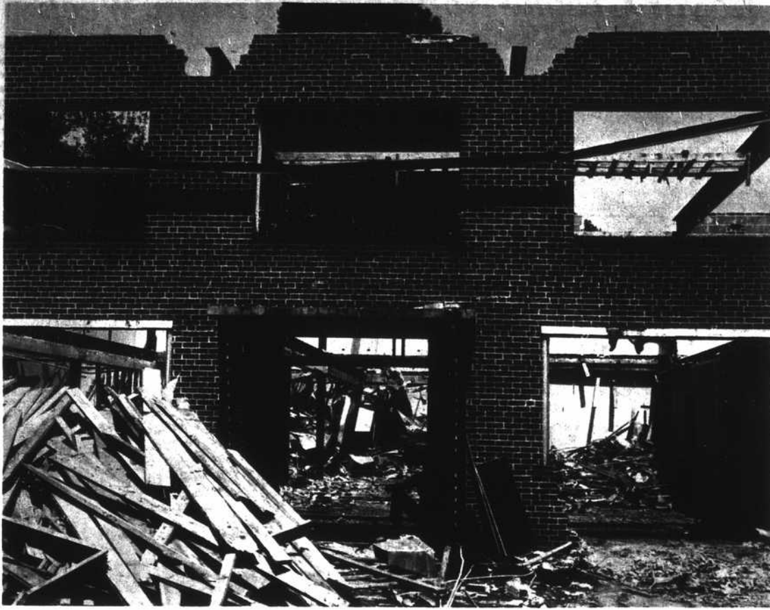
OLD BOOKSTORE COMES DOWN—Appalachian's old bookstore erected in 1934 was being demolished this week to pave the way for construction of a $300,000 split-level structure which will house facilities for merchandising, storage and book rentals.
