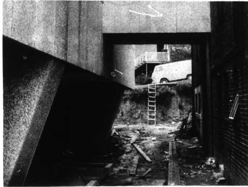
Most Boone residents haven't seen this side of the new court house yet. This is the back of the new building being built on West King Street and at the top of the picture is a passageway leading from the county jail to the new 400-seat court room. A retaining wall will be built against the dirt bank in the background for support. Sidewalks will be added around the new structure to complete the project in early November.
