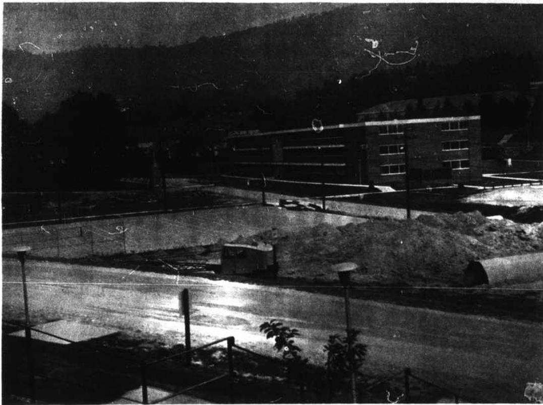
ON THE BOONE THOROUGHFARE route, a drainage pipe almost large enough to be mistaken for a student underpass is being installed (at left in picture). The large classroom building is Edwin Ducan Hall, which is north of the midway mark in the new traffic route. This is the point so long dis-
