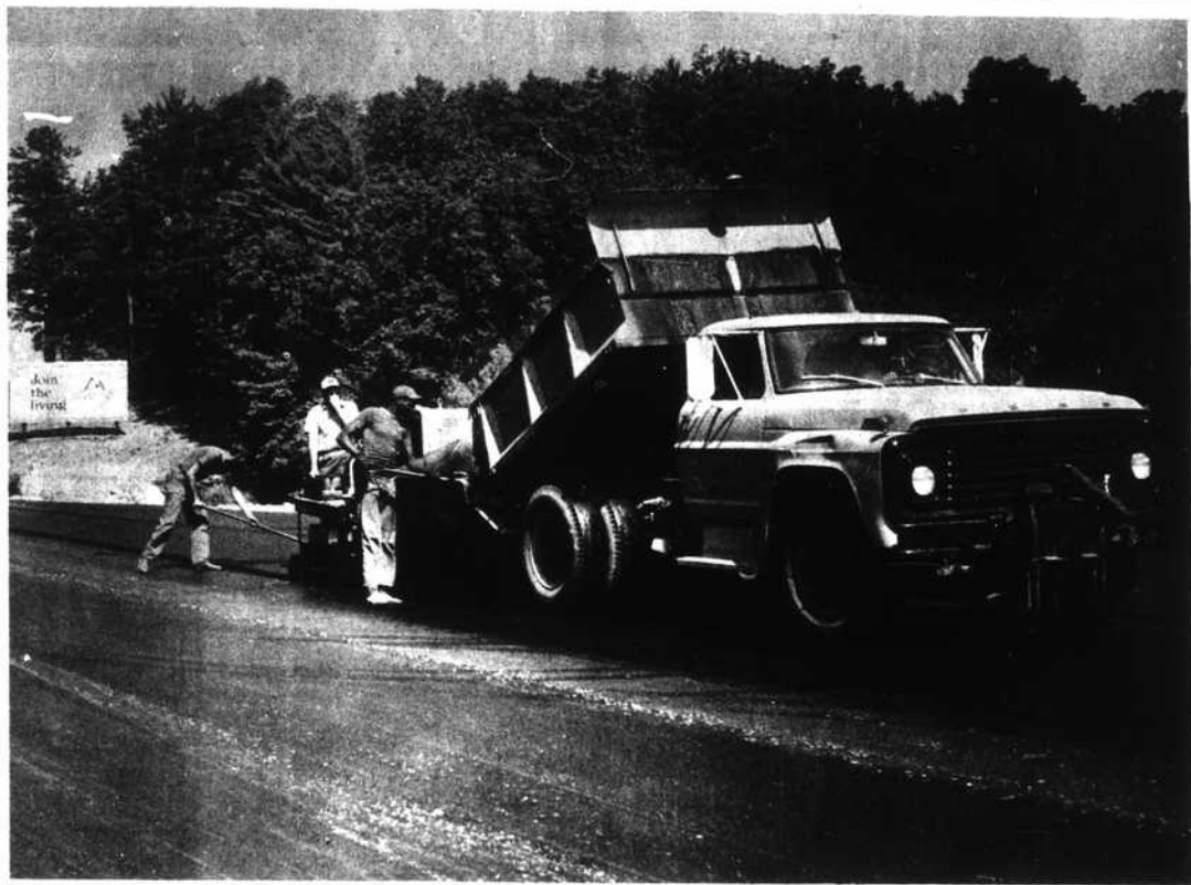
HIGHWAY DEPARTMENT EMPLOYEES put down the black-top on a section of the highway between Blowing Rock and Lenoir. The heavily-traveled road is being widened to three lanes at several points in order to relieve auto-truck congestion.
