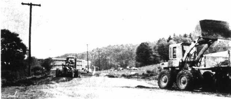
BULLDOZERS AND SCRAPERS speed the Faculty Street improvement project (Boone Thoroughfare) along. Work is now just past the west end of Duncan Hall on the Appalachian campus. The east end of the project at the ASU athletic practice field is paved and usable. The project will go to Water Street where traffic will be turned back to King Street. (Staff photo)
