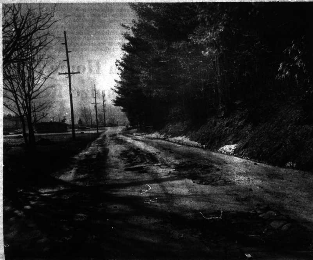
PAVEMENT PROBLEMS—Regular weekend snows and freezing temperatures have ripped and torn the pavement on many Boone streets and scenes such as this early morning shot down Faculty Street are not uncommon in the area. Town Hall says that it will cost a "considerable amount" to restore the streets to proper condition. Damage to this particular section of pavement
