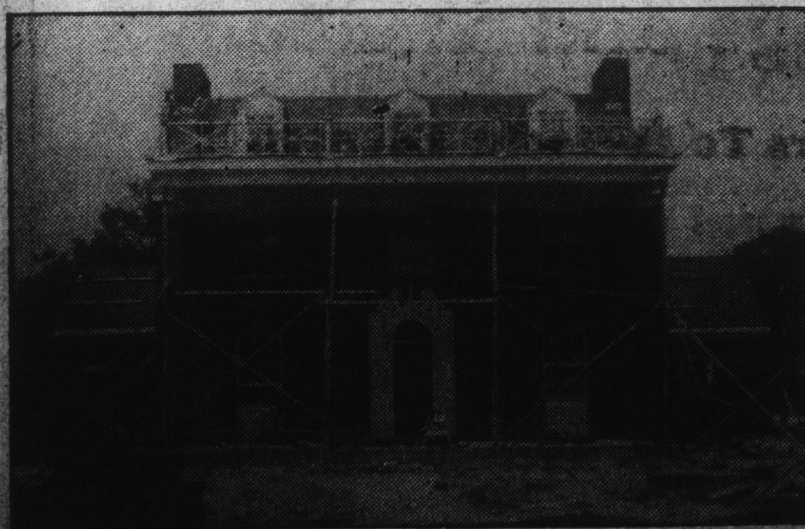
The handsome residence of A. G. Byrum nearing completion, which is being built by the firm of Norris & Hatten, custom contractors, who have built a large number of fine homes in Edenton and the Albemarle section.
