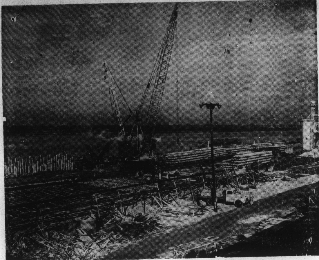
STATE PORT AT WILMINGTON . . . Men and machines lend mutual aid in the state's $5,000,000 port development on the Cape Fear River. To the right are giant reinforced concrete piling over 60 feet long soon to be sunk into the river's bed as foundation for "apron" and terminal buildings. Mixed concrete is forced through elevated pipeline in foreground by vacuum method while to the left are piling in final resting place.
