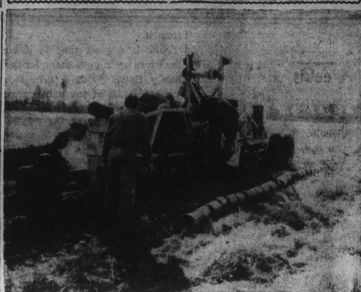
Above is pictured tile being laid on the farm of Carroll Byrum, where six-inch tile is being installed to drain in a field of fall fescue. Mr. Byrum is receiving ACP assistance in carrying out this conservation practice of his soil and water conservation plan.—(Photo by James H. Griffin).
