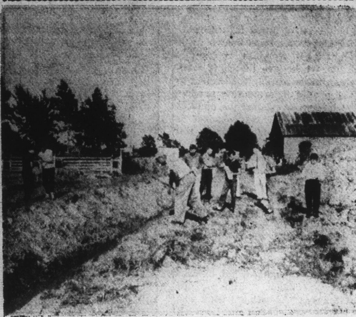
Boy Scouts of Edenton Troop No. 156 are shown above assisting the Albemarle Soil Conservation District with a recent conservation project. They seeded Kobe lespedeza on the berm area of a newly constructed open ditch on the farm of L. H. Haskett on Paradise Road. By seeding lespedeza beside the ditch, the Scouts are helping to control erosion along the ditch. Vegetation slows down surface water during rains, preventing silt from filling the ditch. Gene Ward, local Scout leader, and G. A. Conner, SCS conservation aid, assisted the boys and explained this phase of soil and water conservation. Projects such as this with Scouts is one of the goals this year for the N. C. Chapter of the Soil Conservation Society of America and the local soil conservation district. Boy Scouts earn merit badges as well as learn about the conservation of our nation's resources. John Marshall and Jerry Yarborough of Edenton Troop 156 are now earning their Soil and Water Merit Badges. James H. Griffin, Soil Conservationist, is their advisor in this phase of their Scouting. In the picture, left to right, are: Freddie Ferguson, Bobby Stokley, George Conner, SCS Conservationist aid, Mack Wright, Boots Lassiter, Roland Tolley, Gene Ward, Scout Advisor, Jimmy Dail and Walter Holton.
