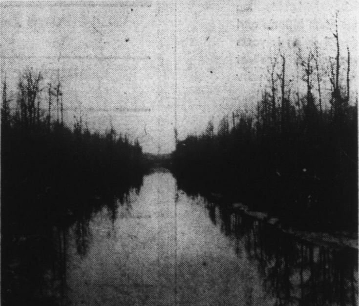
Pictured above is the main channel of Pollock Swamp Watershed near the lower end after completion. This project includes about 21.5 miles of main and lateral ditch construction. A travel way will be established along the edge of the channel for access and maintenance.—(Photo by Sam Cox)
