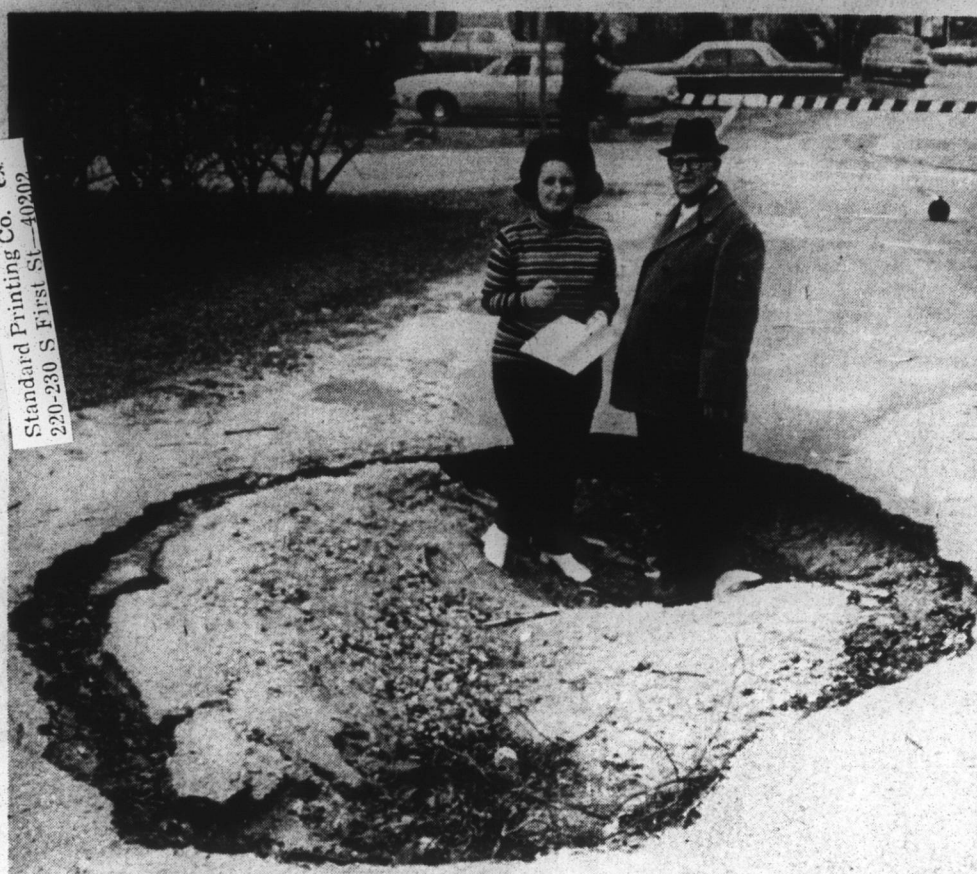
Crisis In Columbia — Deterioration of the sewerage system in the Town of Columbia has caused streets to cave in, shut-down of the treatment plant, a threat to the water distribution system, as well as threatened closing of the hospital and schools. Julian L. Poston, town manager, is shown here with Miss June Myers of Albemarle Regional Planning & Development Commission in one of the holes caused by the problem. ARPDC is assisting in securing federal assistance for the town. (More pictures on Page 1-B).
