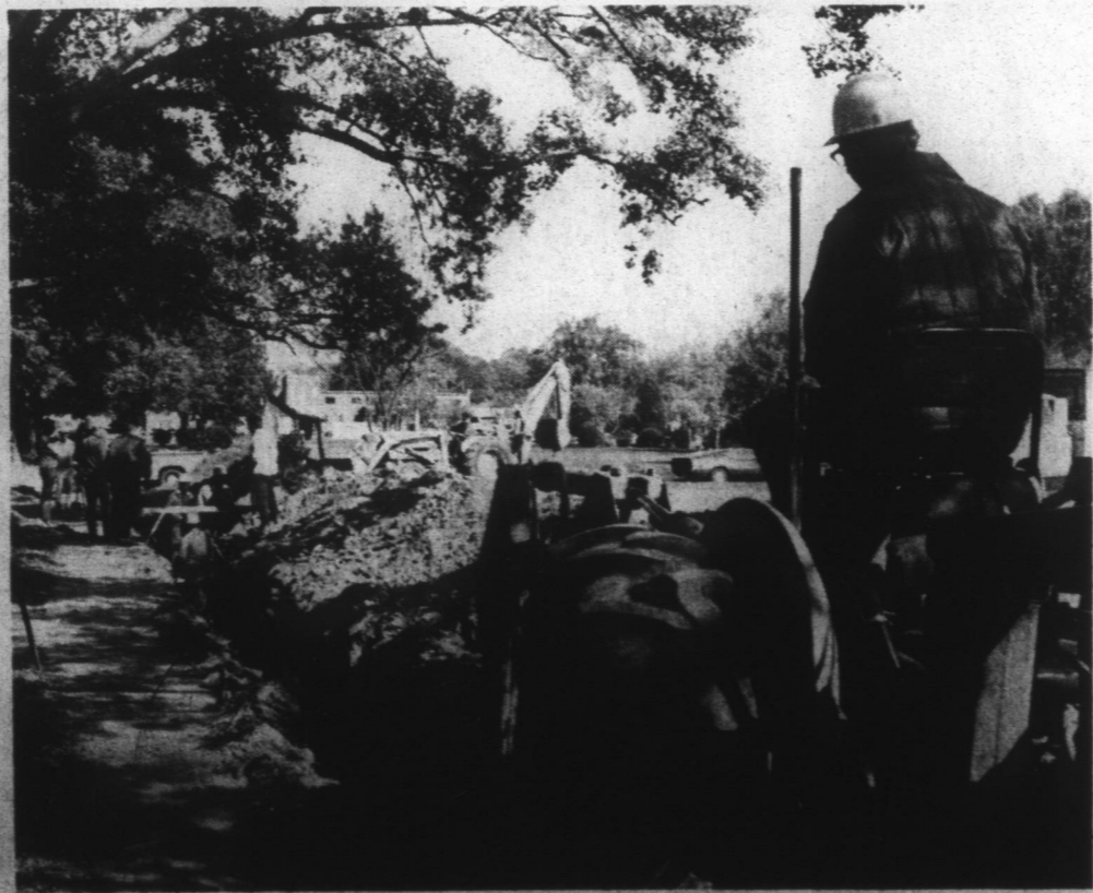
already been installed. The other pictures shows workmen with the State Highway Commission installing a new storm drainage pipe along North Broad Street, near Holmes High School. The new drainage system is expected to halt periodic flooding in the area of Habit's Motel.
