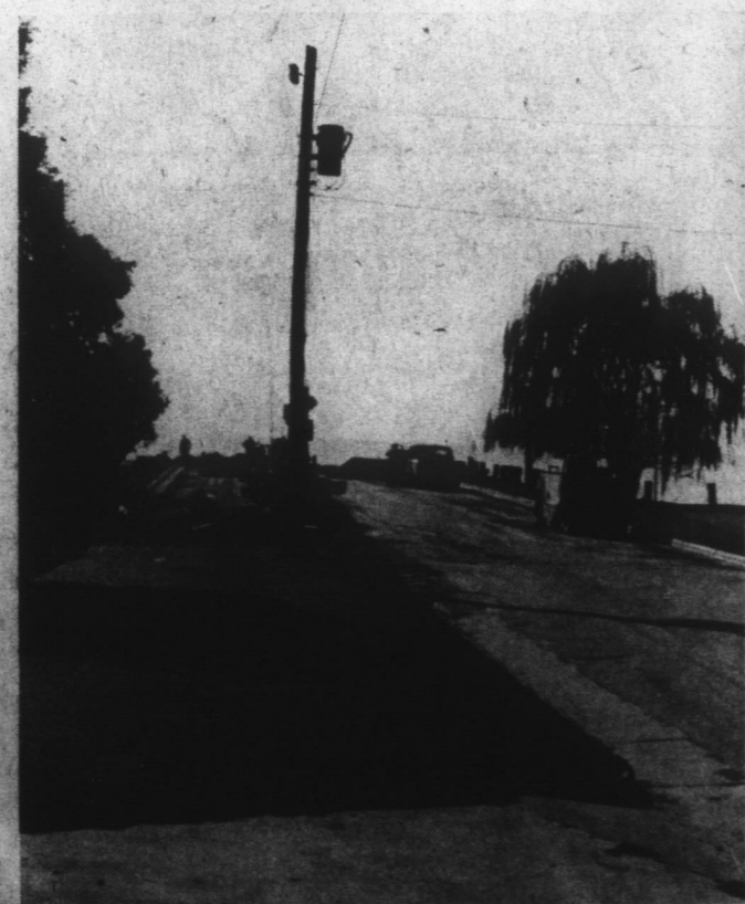
IMPROVEMENTS BEING MADE --Workmen this week were busy making improvements in two sections of Edenton. At left, Rose Brothers workmen are shown preparing to pave the lower end of South Broad Street which will provide paved parking at the Barker House Visitor Center-Museum. Curb and gutter has
