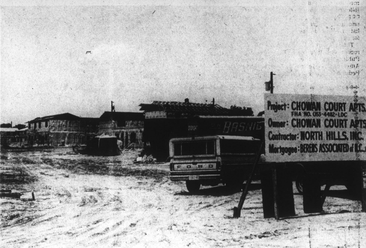
CONSTRUCTION UNDERWAY —Currently under construction is the 50-unit Chowan Courts Apartments, contracted by North Hills Inc. It is not known when all units will be completed in the privately owned, government subsidized project, but several of the apartments are scheduled to be ready for occupancy by the end of June. Construction began last October but inclement weather has hampered completion.
