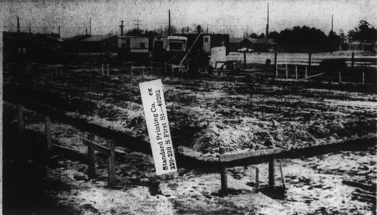
NEW CAFETERIA BEGUN —The initial phase of construction on the new D. F. Walker School Cafeteria has begun with staking out the grounds and digging foundation trenches. The $216,000 facility will be located behind the gymnasium, adjacent to the elementary grade buildings. It replaces the lunchroom which was destroyed by fire last year.
