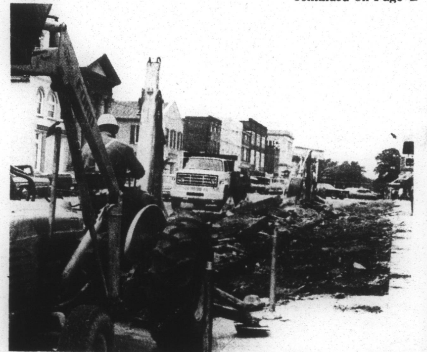
WORK GOES ON —Work on the downtown Edenton improvement project began in the block between King and Water streets this week. Crews were taking up curb and guttering as well as a portion of the sidewalk, as is shown here, while others followed with conduit for underground wiring. Putting down the brick sidewalks will begin June 16. W. B. Gardner, town administrator, said the brick work has been delayed to allow workman to get as many tree wells, conduit and curb and gutter in as possible.
