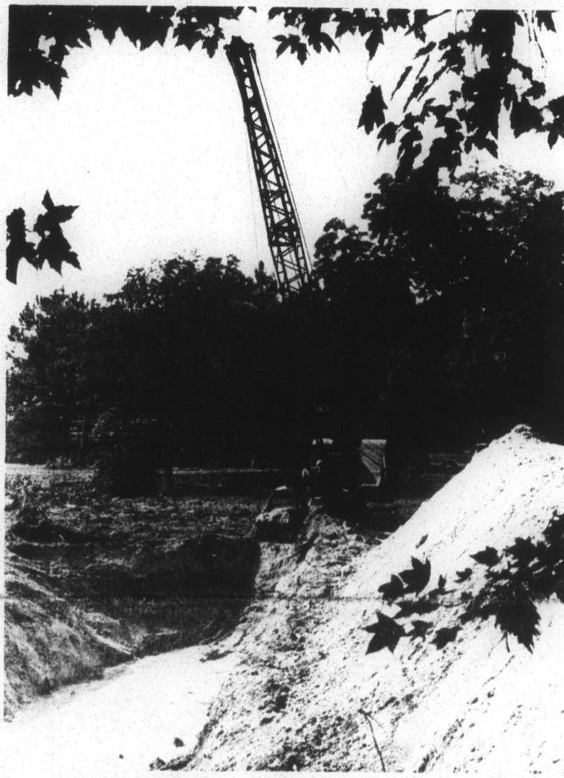
PREPARE FOR DREDGING —A dragline is shown here as work is underway on a dike at the site of where spoil material will be placed from dredging of a channel in Pembroke Creek. Actual dredging on the Corps of Engineers project is scheduled to begin Monday.
