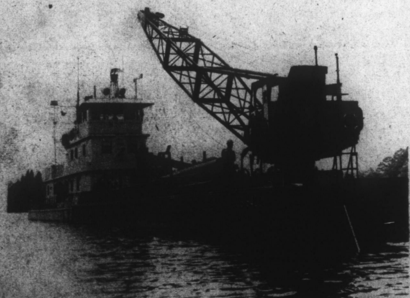
CLEANING UP—A U. S. Coast Guard barge equipped with cranes was involved in cleaning up hazardous snags loosened by the recent dredging of Pembroke Creek. The dredging and subsequent clean-up has deepened the channel in the creek leading to Edenton Marina.
