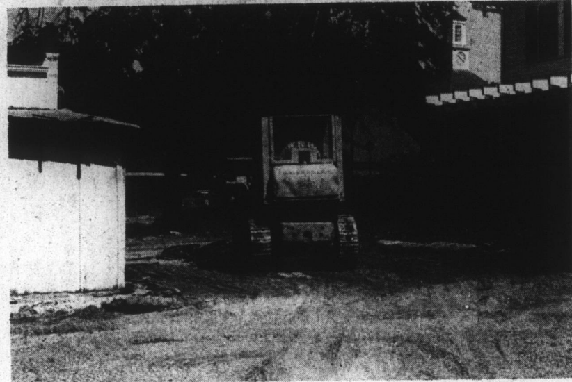
DEMOLITION STARTED — Demolition on the site of the Chowan County Courthouse-Jail complex began in May at the corner of Broad and Queen streets. A BP service station on the corner was the first structure to fall.
