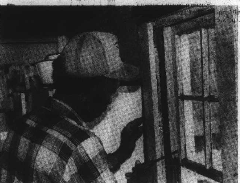
WEATHERIZATION —James Jackson, EIC carpenter, is making a window air tight at the home of Calvin Moore, 220 W. Carteret Street. The work is being done by EIC as part of the Dept. of Energy's Weatherization Program.
