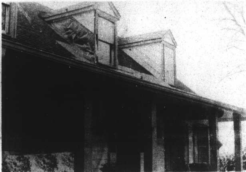
HOUSE DAMAGED—The home of attorney Max Busby recently sustained major fire damage due to a short in a water pipe heater tape. Dormer windows are temporarily sealed against the weather by plastic and plywood while holes in the porch ceiling gape open where firemen gained access to the fire. Damage was estimated at $50,000.
