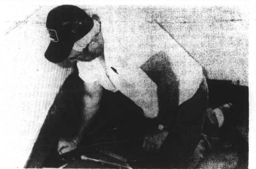
NEW CARPET INSTALLED —Jake Dunlow of Carpet and Appliance Plaza tightens new carpet that the company is installing in the remodeled Chamber of Commerce offices.
