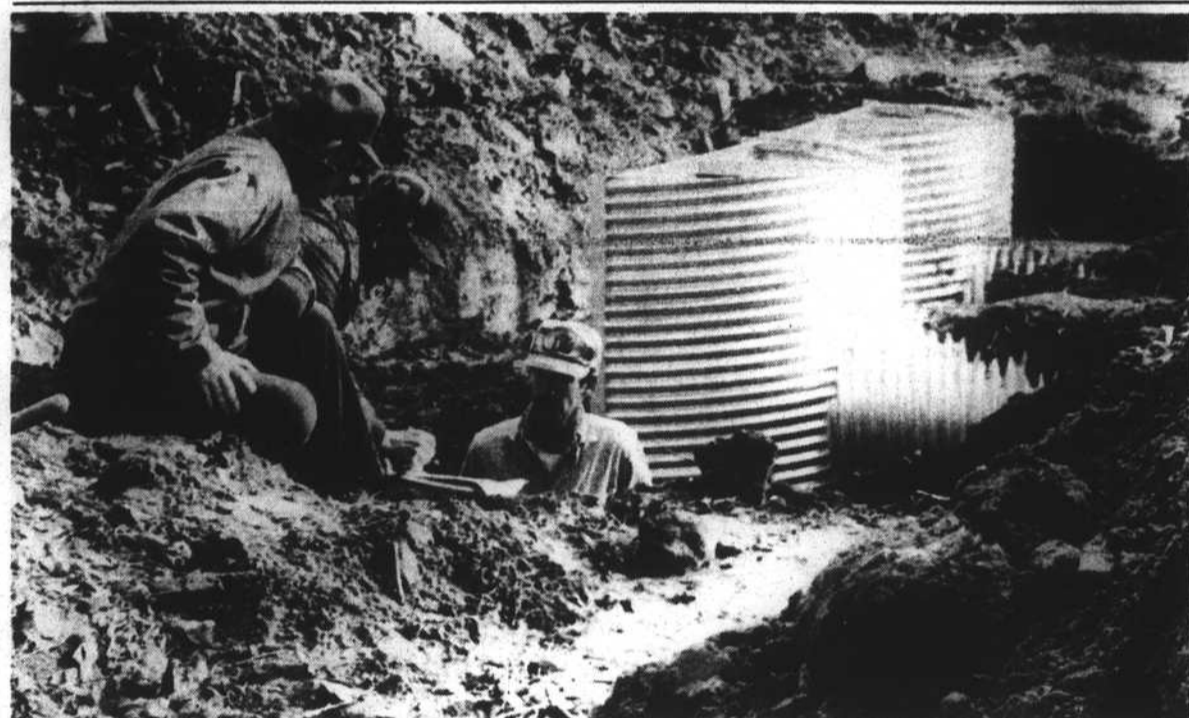
DISCUSS PLACEMENT—Jimmie M. Parrish (left) and son, Frankie (right) discuss with SCS technician Stanton Harrell the placement of four flashboard risers on Parrish property. The drain pipe is 30 feet long, 42 inches in diameter and the risers are six feet high.
