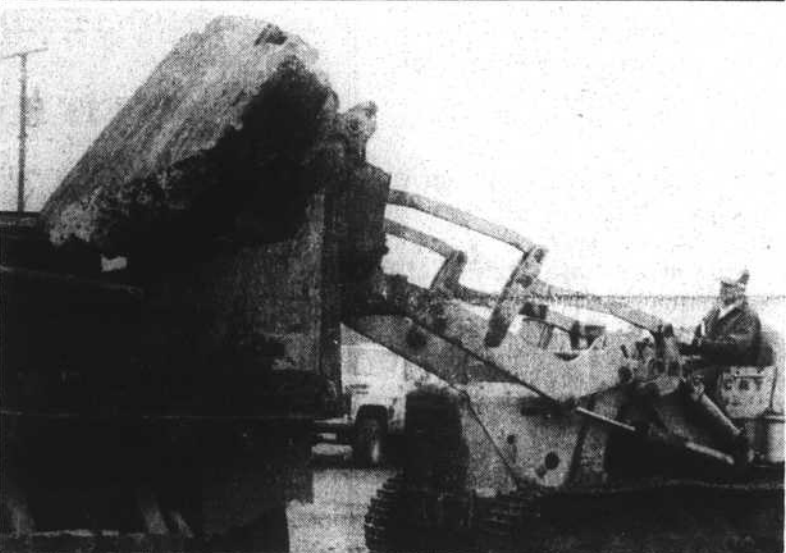
UP AND IN —A piece of heavy concrete rubble is loaded into the steel bed of a truck Thursday. The use of heavy equipment such as this was donated in the cleanup of the Rocky Hock Grocery debris.
