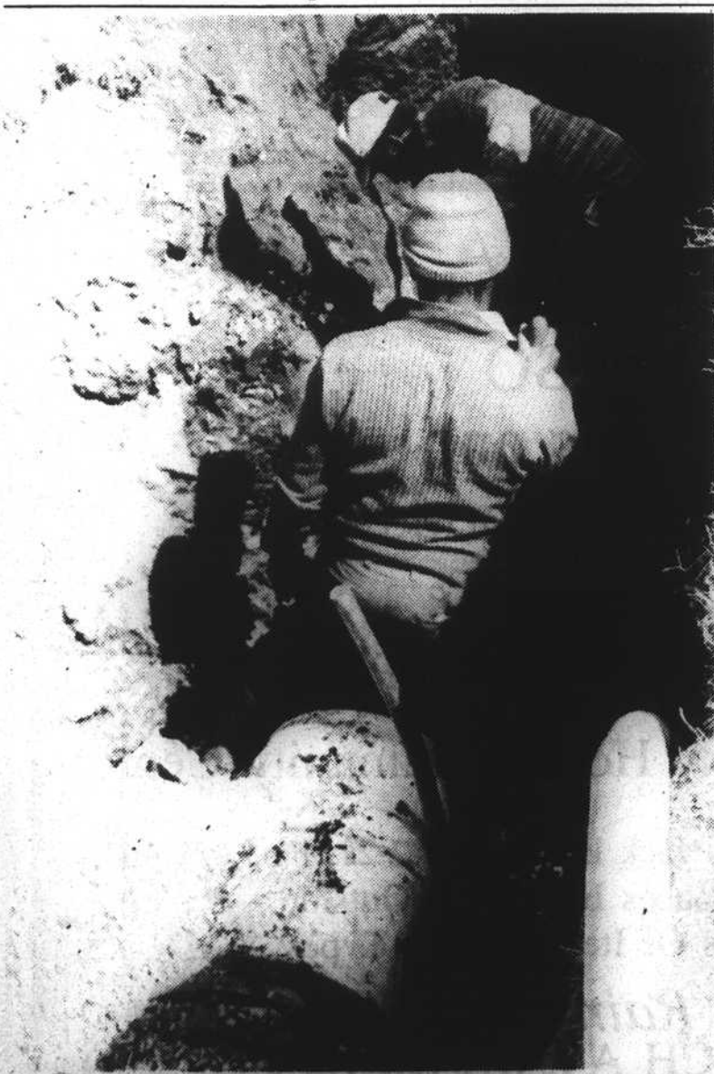
NEW SEWAGE LINES —Workmen were busy installing new sewer pipes at the corner of Granville and Water Streets this week. Residents have had to detour as some streets west of Broad have been blocked off to allow for the installation of the new lines which will connect with the waste water treatment plant to be completed early next year.
