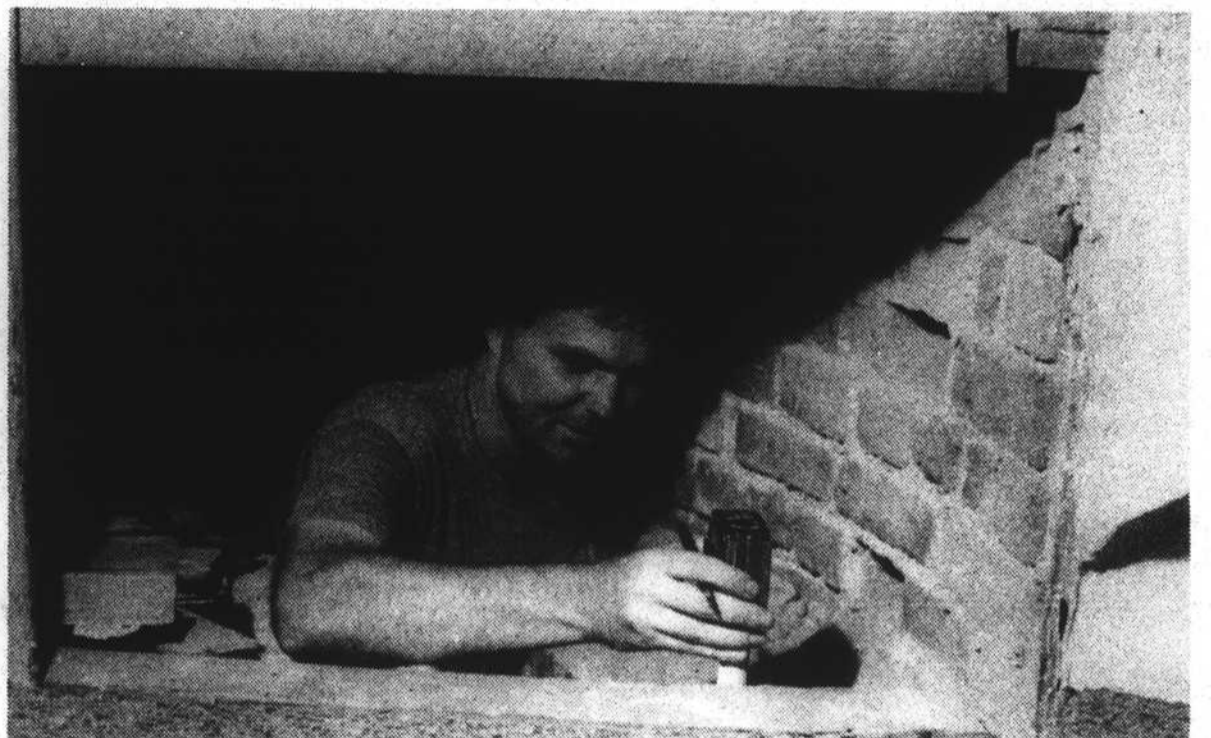
HISTORICAL DETECTIVE —A physical survey of Chowan's 1768 courthouse allowed a research team from Colonial Williamsburg to get a close look at the structure's construction. A researcher is shown taking measurements beneath the judge's rostrum. A team member pointed out the uniqueness of the Edenton landmark as "a working building and not just a museum."
